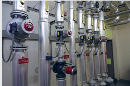
Five circulators. One circulator is a complete Motor Driven Unit consisting of VFD, motor, pump (Source: Impact Energy, 2016)
